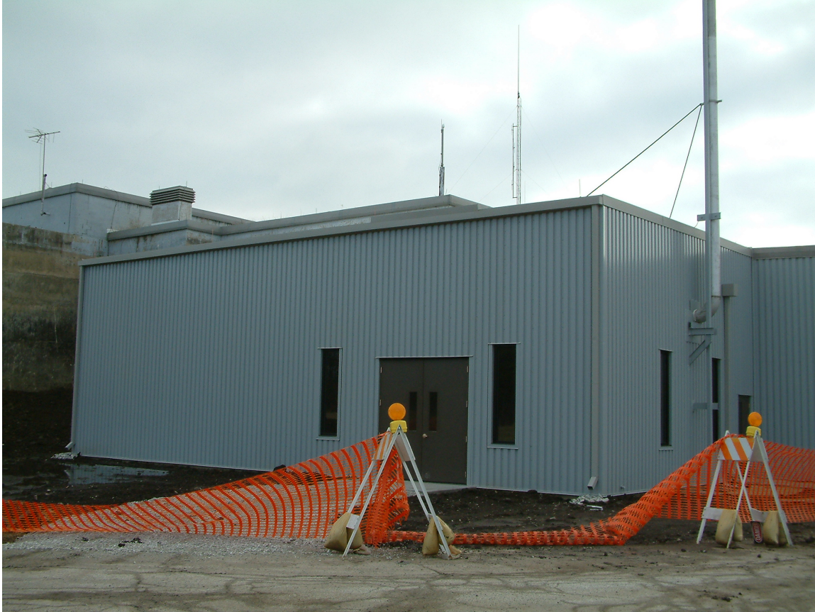
Fig. II-8. Building addition for the CARIBU facility. The addition is funded as a separate laboratory project.
