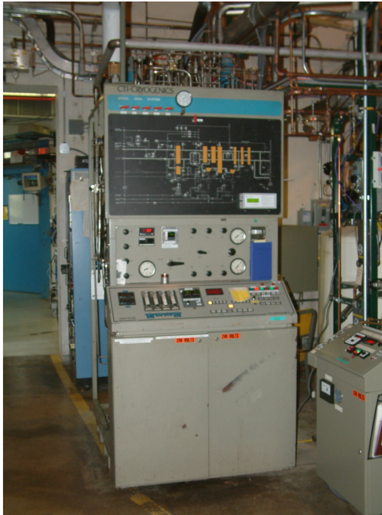
Fig. II-5. CTI Model 2800 – 300 Watt liquid helium refrigerator shown after installation in the ATLAS facility.
